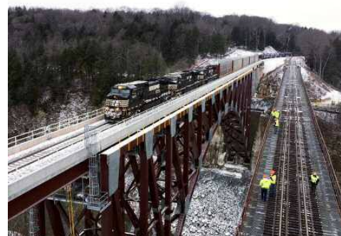
At 2:20 P.M. DEC. 11, NORFOLK SOUTHERN GENERAL MERCHANDISE TRAIN 36T BECAME THE FIRST TO CROSS THE NEW PORTAGEVILLE BRIDGE
